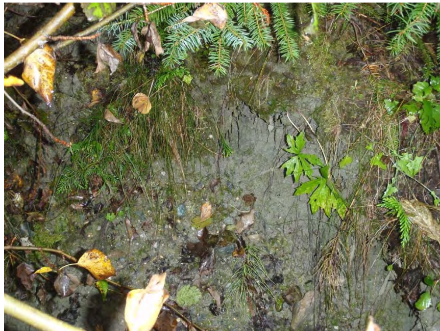
Photo 2. View of minor erosion on left side of stilling basin at redirection where ephemeral stream enters. No work warranted at this time.
