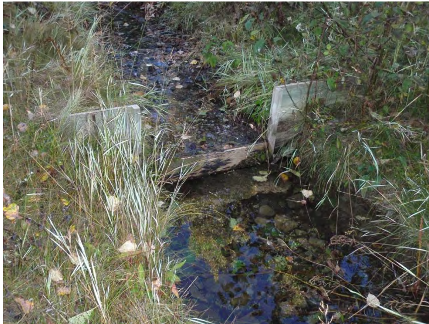
Photo 24. View of area of minor channel erosion in lower Segment X, immediately below the concrete and wooden weir located just upstream of the inlet of the culvert under Johnson Lake Road. Eroded channel banks should be armoured to help prevent future erosion. Water currently flows under weir. Weir should be relocated or repaired, as required.
