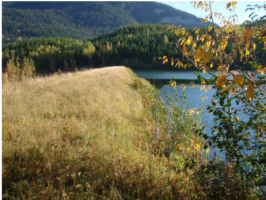
Photo 10. View of upstream face of tailings dam. Eroded and undercut portion at waterline shows no significant change since the last inspection. Note cattails planted along the waterline to help reduce wave action erosion of the upstream face.
