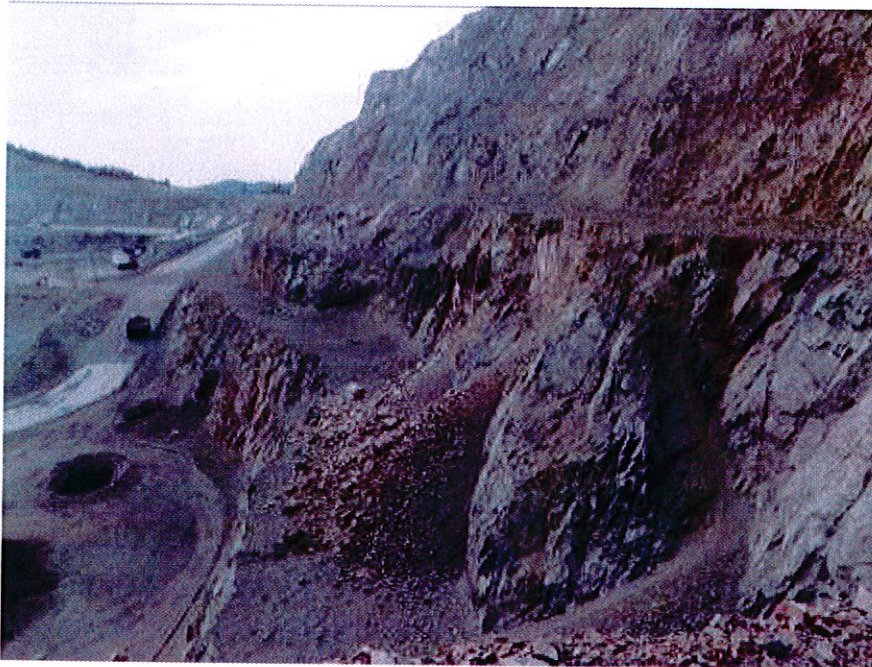
Photo 4: Accumulation of rockfall on 1048 bench poses a rockfall hazard to persons below. Note that drillers were recently working within about 12m of the toe and a pipe line is located along the toe on 1024 bench.
