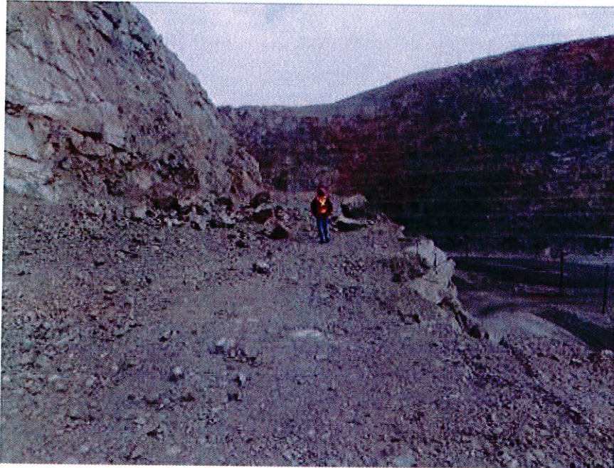
Photo 3: South side of 1072 Bench. Crest break back on geologic structure locally reduces bench width from the planned 12m down to 7m. Note only isolated rockfall blocks.
