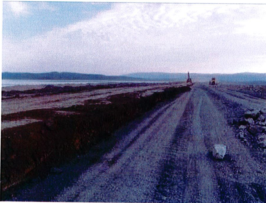
Photo 6: TSF. Stage 8 till and filter construction. To facilitate compaction till is placed at 2:1 slope beyond line then trimmed back.
